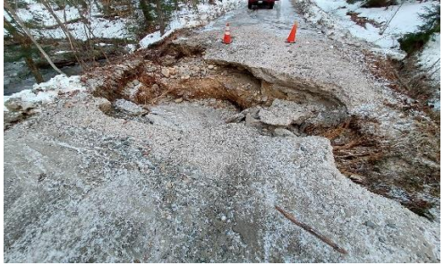
Decker Road Washout
